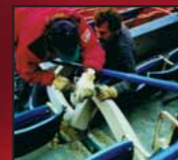
Expansion jointing for civil engineering project (Shae Stadium, Home of Major League Baseball's New York Mets)
